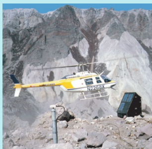
Figure 2: Remote station with solar panels and a GPS antenna Photo Credit: Dan Dzurisin, USGS
